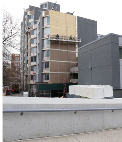
Top: Center pathway within complex to school. Bottom: EIFS being applied over the original ribbed-concrete block. Nov. 2021
